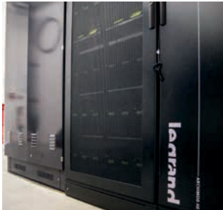
The Archimod 240 kVA ondulator is a modular solution that enables UPSs and batteries to be added as the data centre expands.
