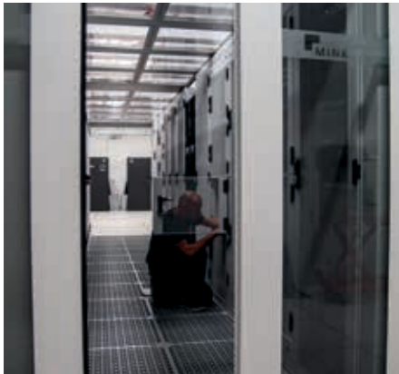
NeoCenter Ouest has the fourth and last version of the Cold Corridor developed by Minkels, which has space for 40 racks.
