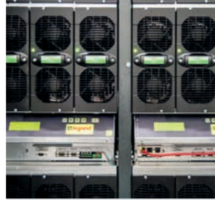
NeoCenter Ouest has the newest generation of UPSs with the Archimod 240 kVA by the S2S company (Legrand Group).
